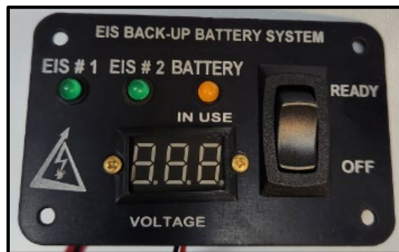
Figure 1: EIS Back-up Battery System Panel
