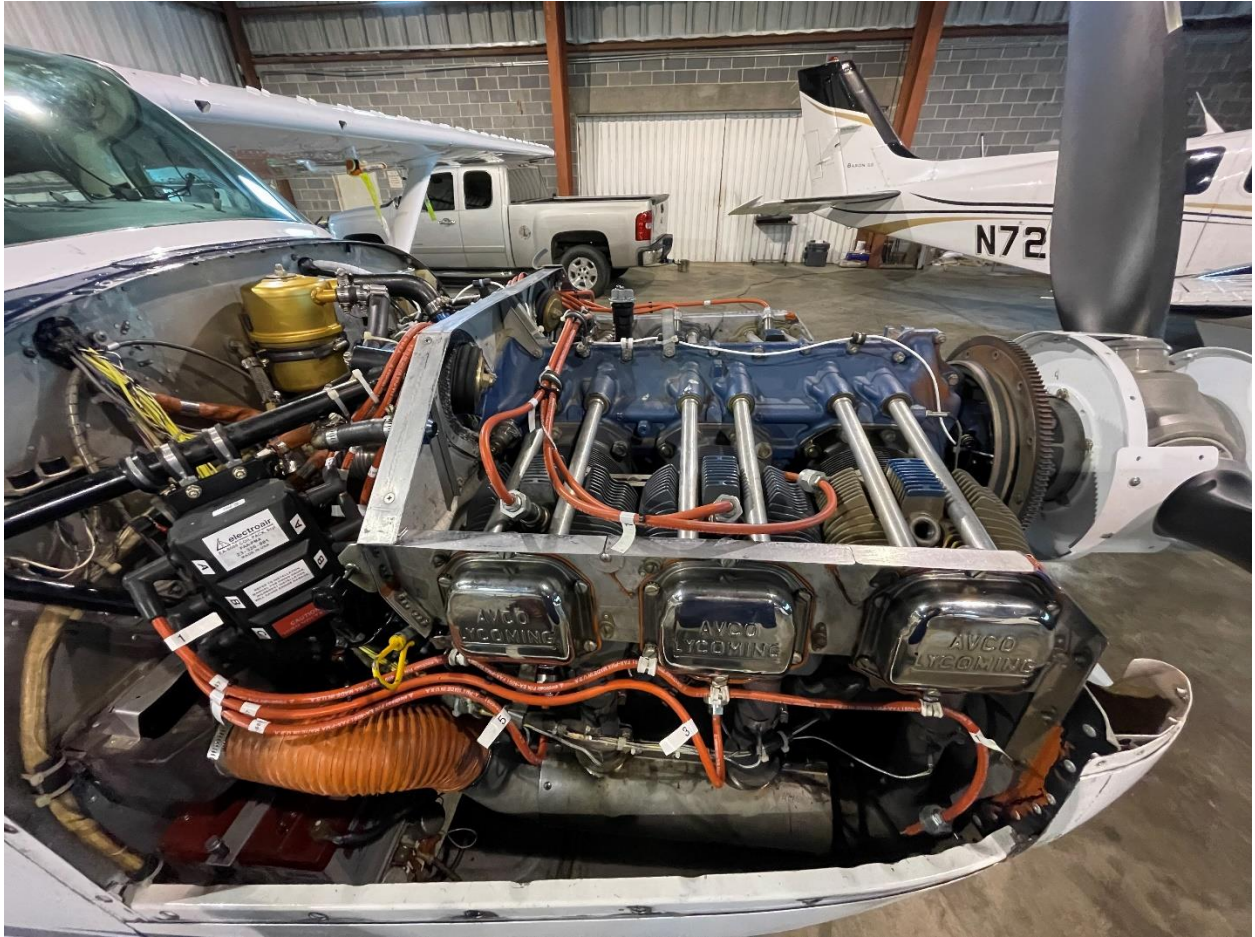
Right Side Installation, Coil and Wires Left Side Installation, Coil and Wires
