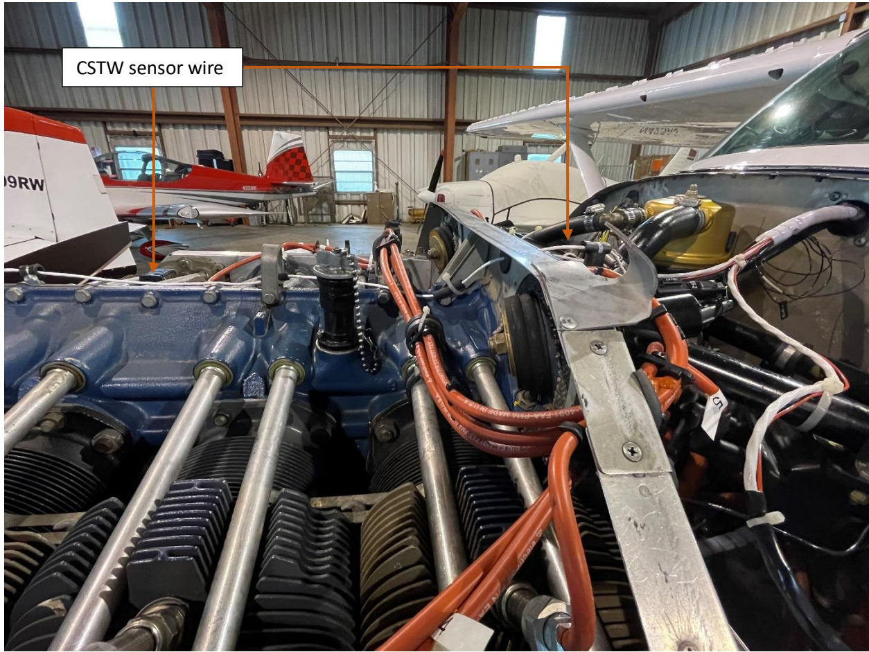
CSTW Sensor routing (white wire) around sparkplug wires
